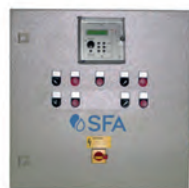
PS2 system box
